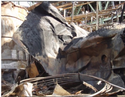
Fig.2 Damaged Tank (View from southwest and zoom in)
